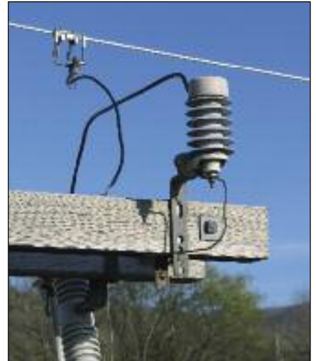
Although a lightning arrester looks like an insulator, its purpose is very different.
